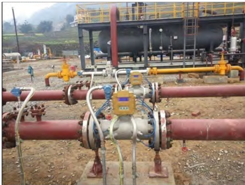
BFUG-200mm PN6.3MPa application for shale gas distribution metering in Ning 201H1 platform in Sichuan gas field
